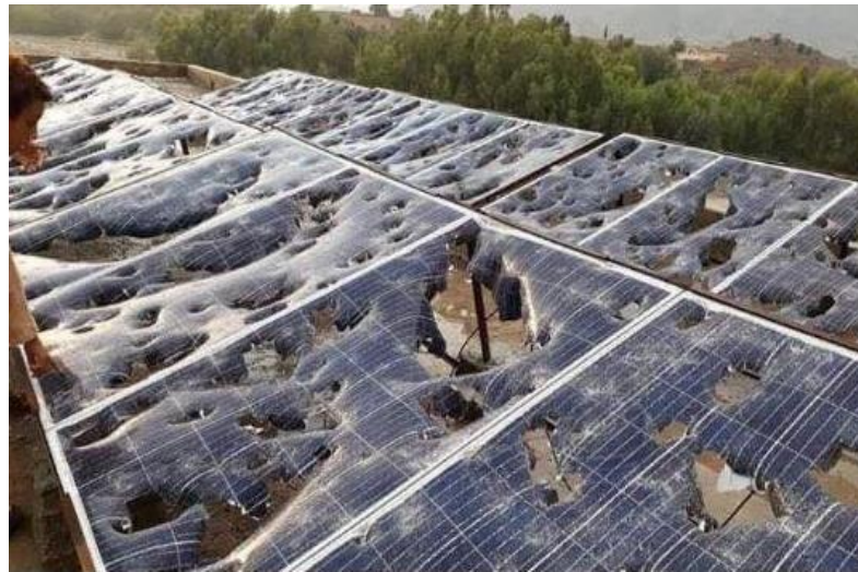
Large-hail damages on solar panels
